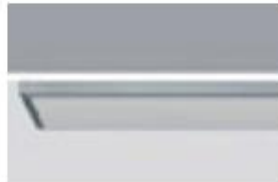
Oberhalb Service APL Above service workstations
